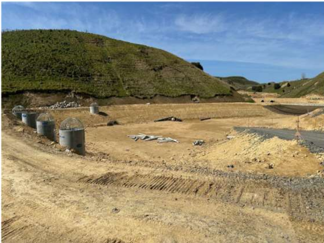
Image 9. Construction of new Area B at Ōmarunui Landfill showing the clay liner, leachate and stormwater catchment infrastructure
