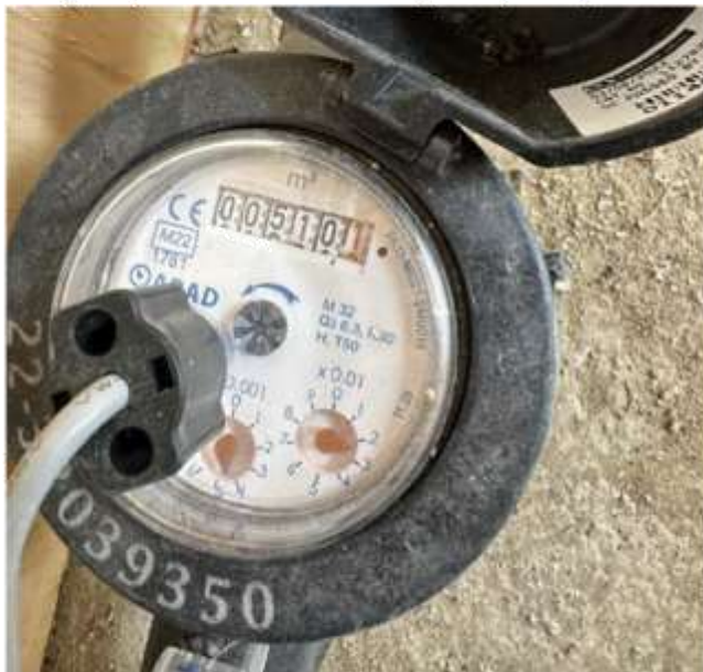
Image 3. An in-line water meter with telemetry ability
