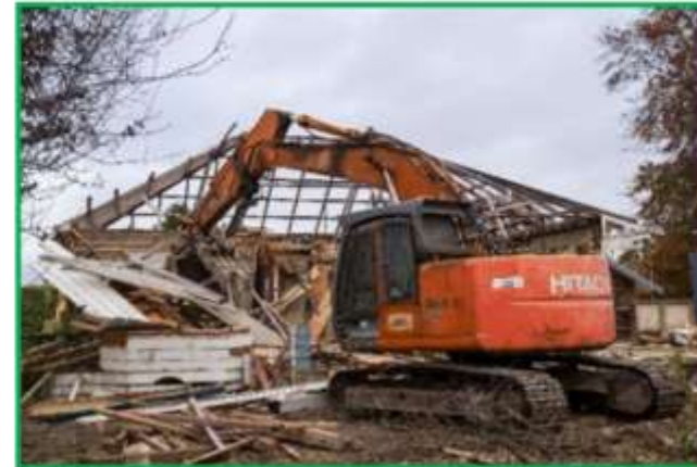
Demolition of the first Category 3 property to go through the process. This property was in Pakowhai.
