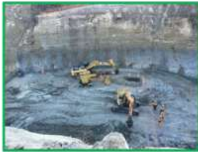
Dartmoor Road slip. Downers construction working at the slip site below Dartmoor Road
