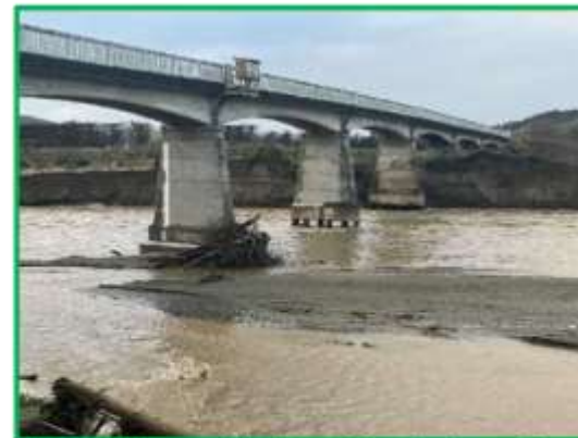
Waipunga Bridge scour during rain events is causing increased scour around pier 5
