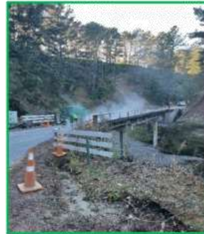
Waikoau Gorge Bridge Fulton Hogan staff working to strengthen the bridge decking
