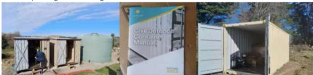
Figure 2: Mataweka marae new water storage and emergency container.
