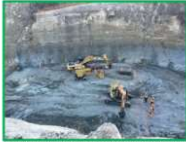
Section in Kereru Gorge site being marked out before soil mixing, 11 June 2024
