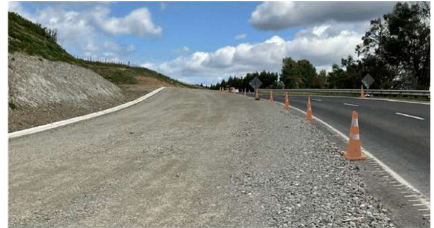
The slow vehicle bay on the Mohaka Ascent is prepared for sealing (top)
