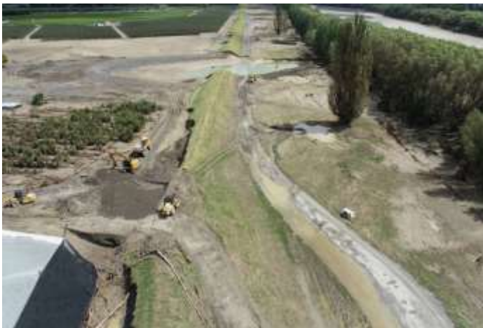
Figure 3: Moteo stopbank breach
