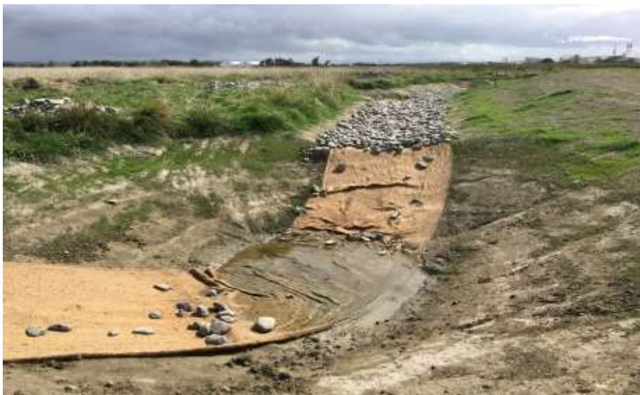
Fig.3: Outlet and fish passage channel 1 of 3 ponding areas.
